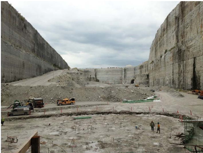
The first section of the McCook Reservoir, holding 3.5 billion gallons, is nearing completion in 2017. The reservoir is the final component of the Metropolitan Water Reclamation District of Greater Chicago’s Tunnel and Reservoir Plan.
