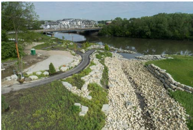
The diversion channel for the Midlothian Creek Flood Control Project in Robbins that the District helped fund is an example of a stormwater partnership project directly supporting municipalities in Cook County to address localized flooding and drainage concerns.
